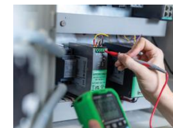
Industrial Automation & Control
